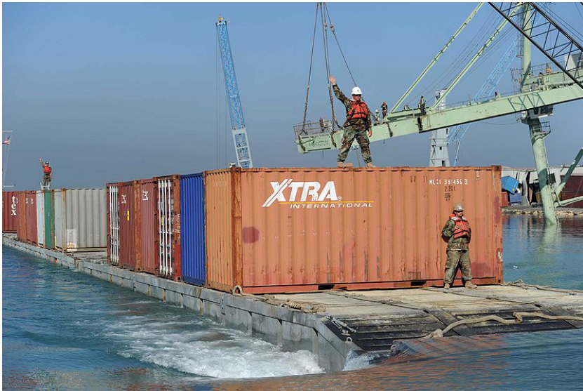
Figure 7: A floating pier
