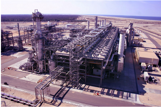
Figure 8: Damietta LNG plant, which is back online with an annual production capacity of around 5 million tons of liquefied gas and the potential for a further increase with an expansion 37
